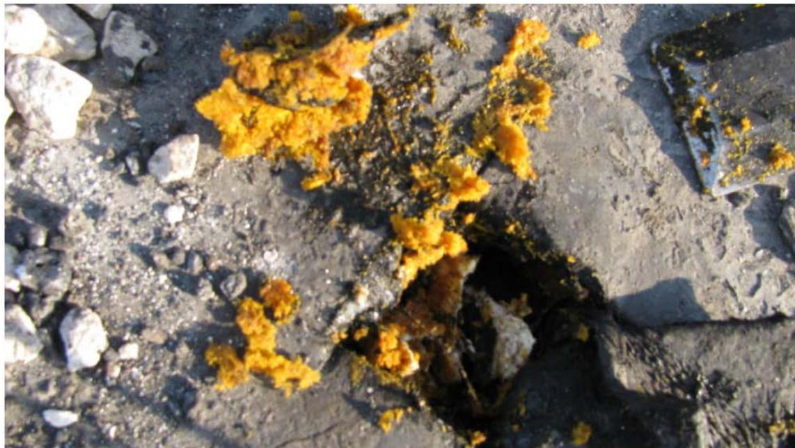
Figure 2 – Evidence of Wet Insulation at J. Don Boney Building
