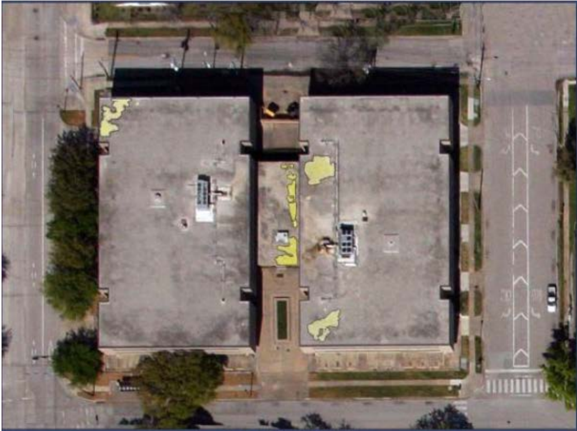
Figure 1 – Infrared Photo of BSC, CIC, JDB Buildings showing Moisture Infiltration
