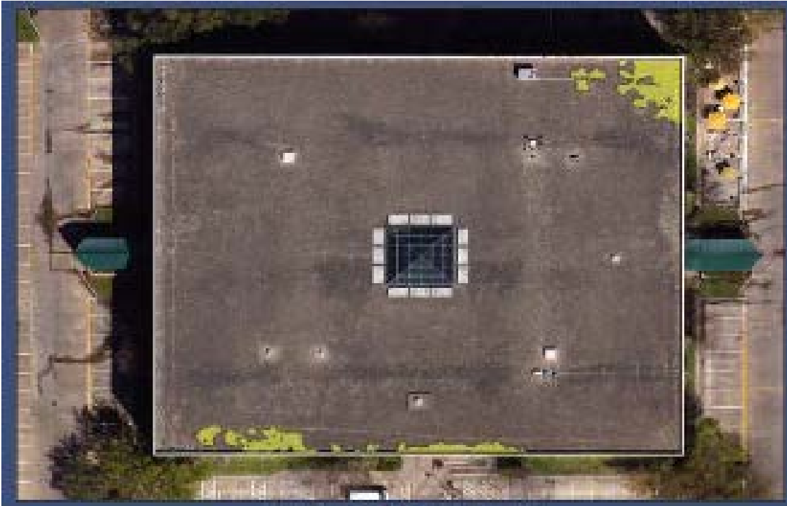
Figure 1 – Infrared Photo of Katy Roof Showing Areas of Water Infiltration
