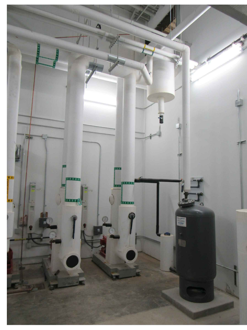
PHOTO: EXISTING CHW PUMPS TO REMAIN
