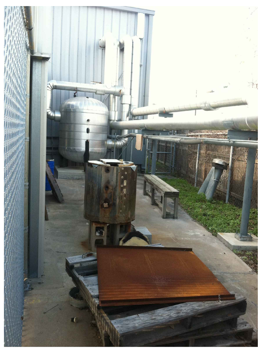
PHOTO: EXISTING VOLUME BUFFER TANK AND PIPING
