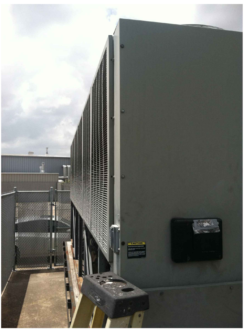
PHOTO: EXISTING CHILLER ON TRAILER
