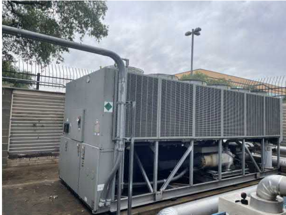
Photo 13 View of an on-site chiller
