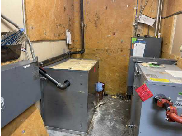
Photo 7 View of on-site elevator equipment
