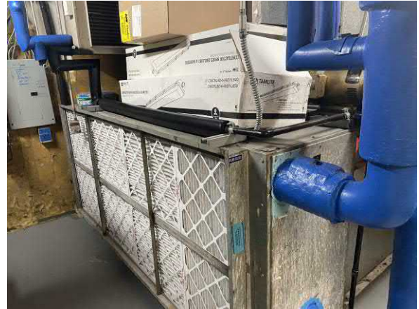
Photo 8 View of an on-site air handler unit
